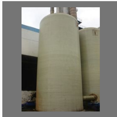
Water Storage Tanks
